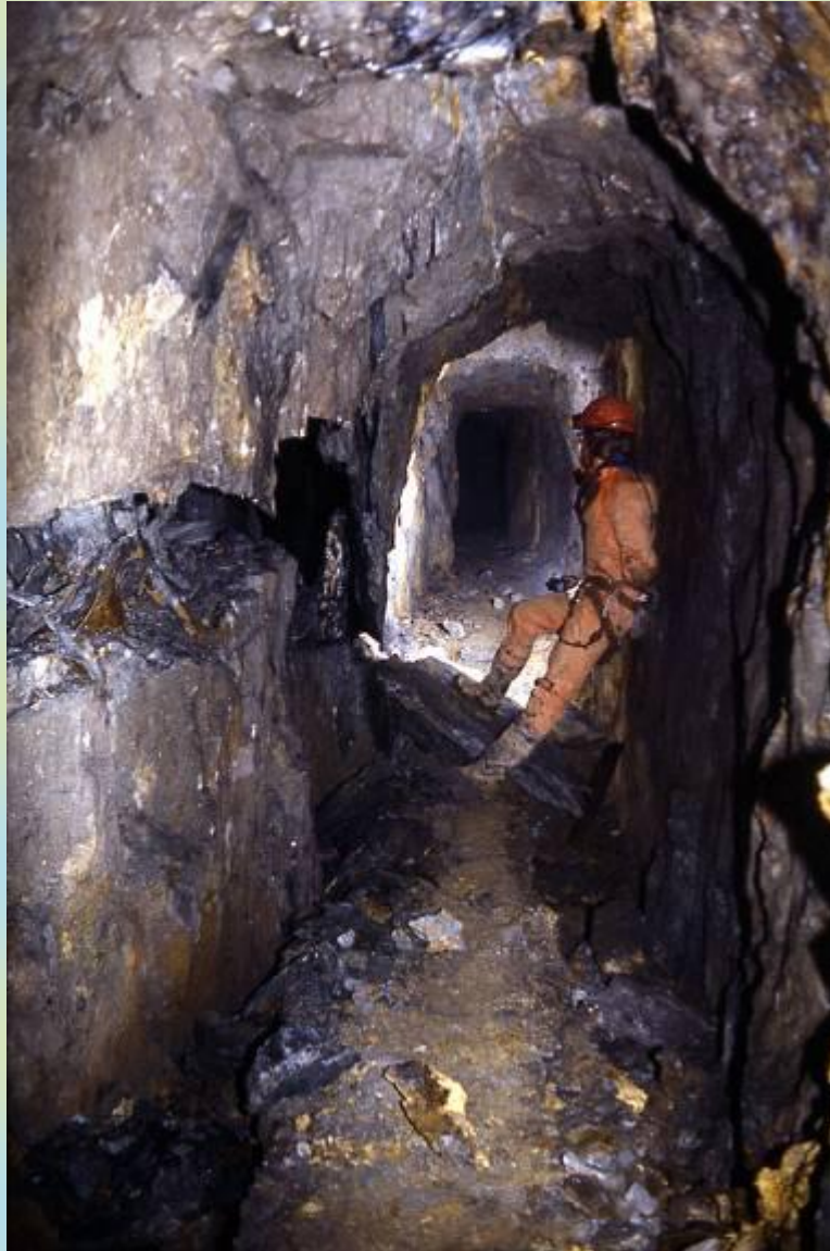
A highly stressed tunnel exhibiting large cracks and fractures in the walls and floor was aptly named "Earthquake Passage." T.L.E. Plan No5.
